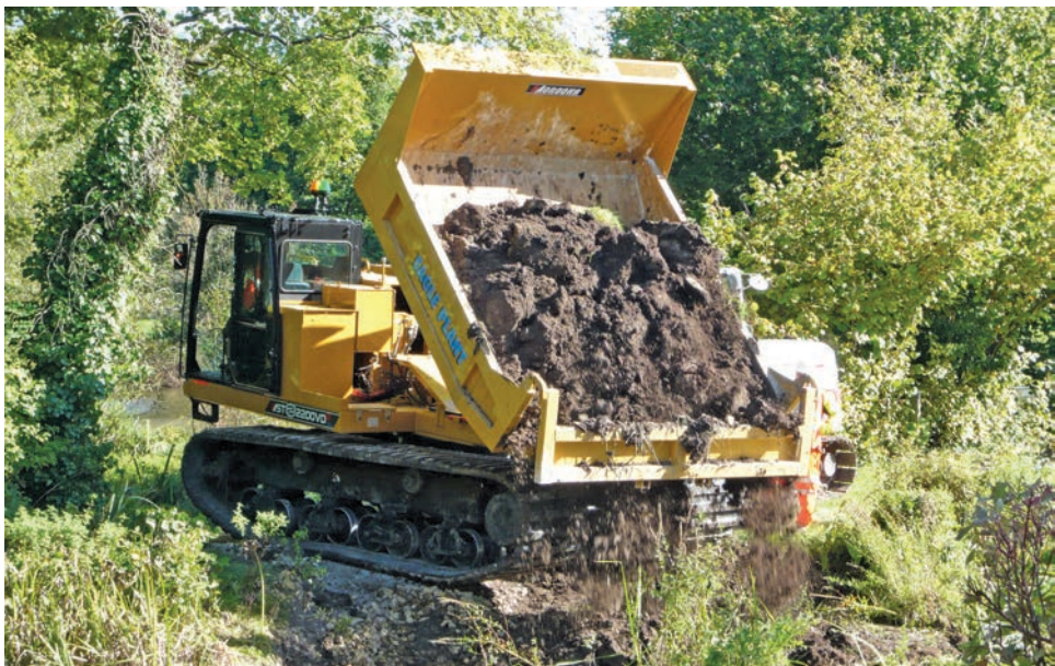
Heavy plant used for infilling the new berms on the Avon – photo by Editor
