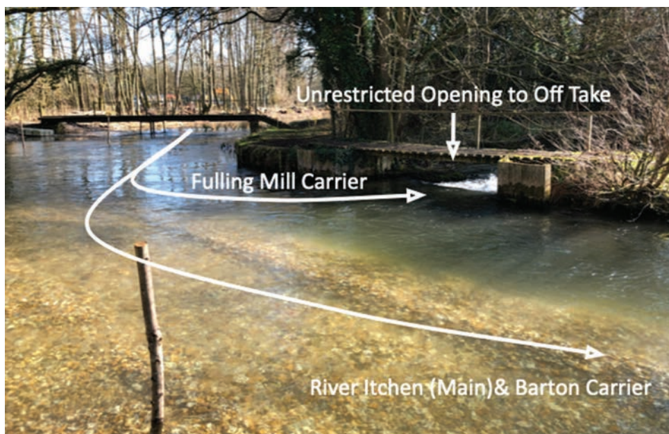
Fulling Mill off-take structure showing flow split
